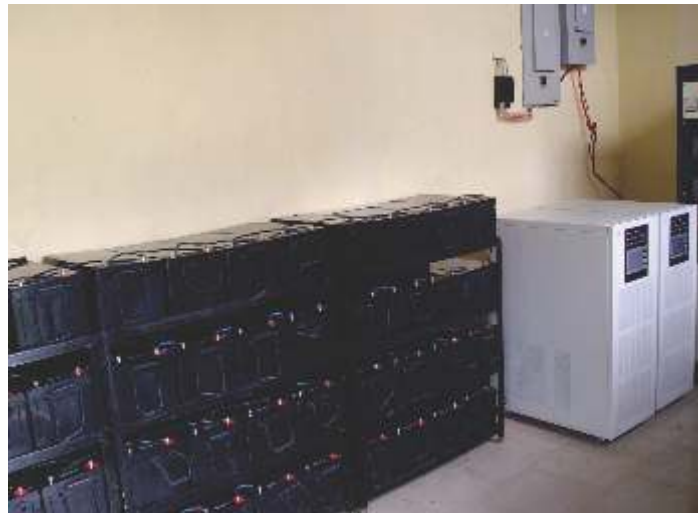
Quintas 60KVA (30kva each) Inverter Installation @UCTH Calabar
